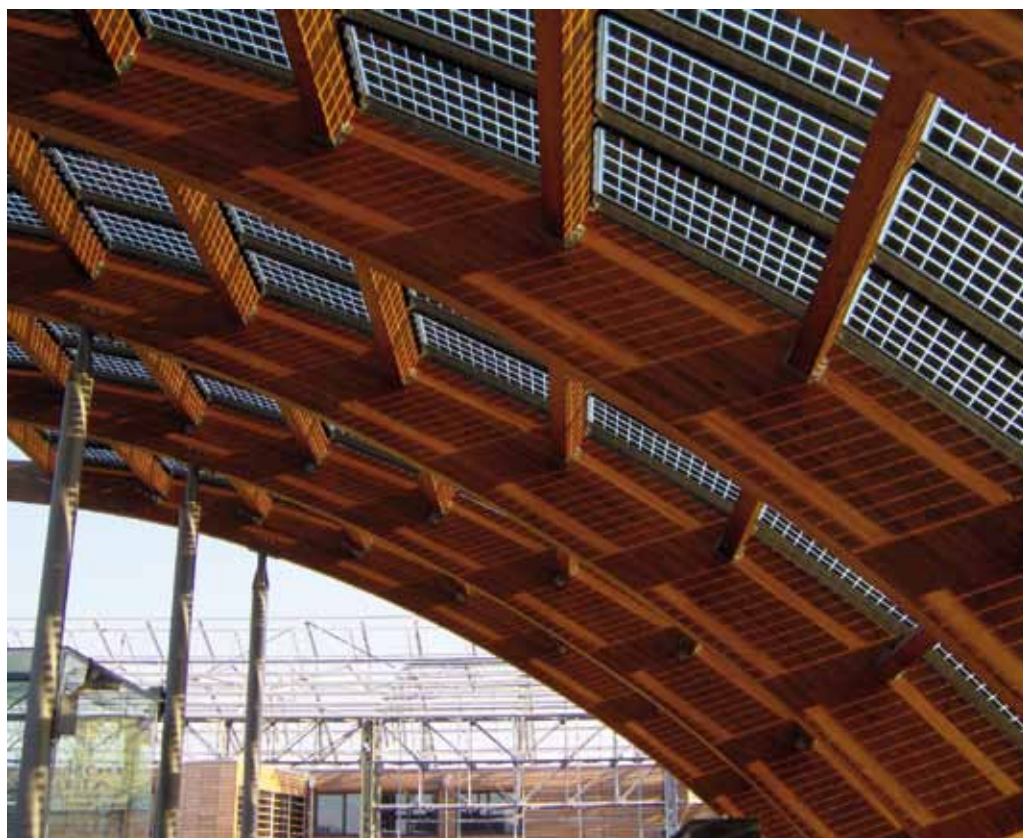
Fotovoltaico integrato Environmental Park (TO)
